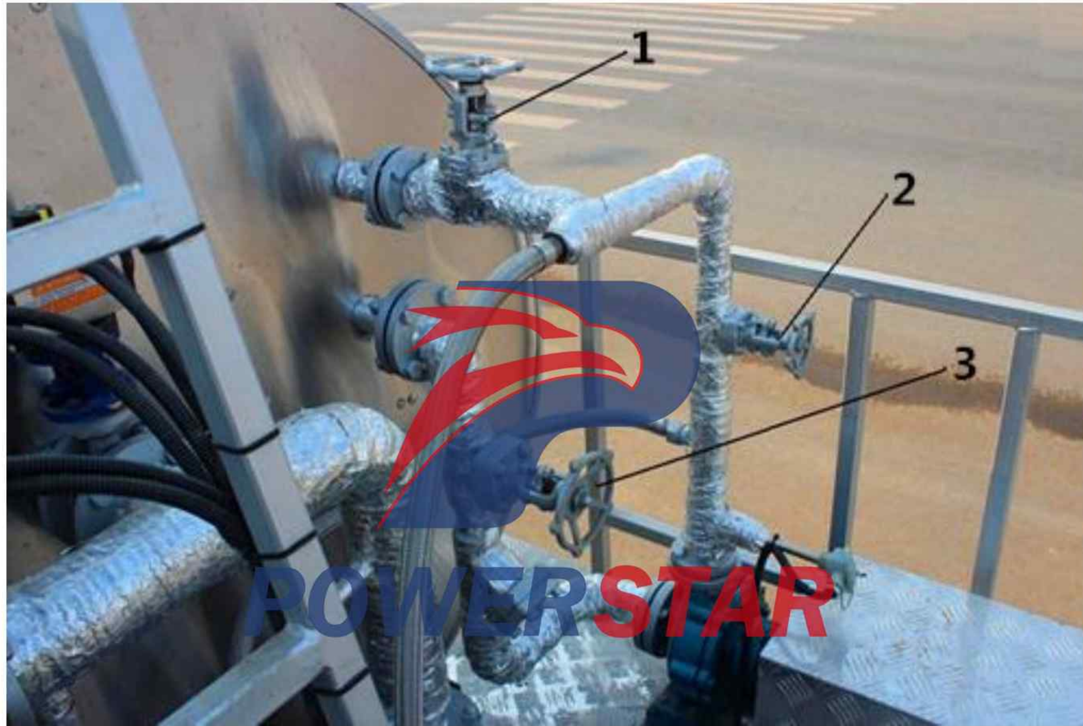
Fig. 11 Heat transfer oil valve
